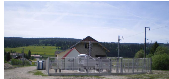
SVC installed in France
