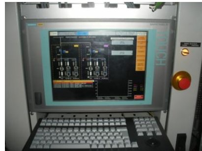
Local control panel PC with SCADA
