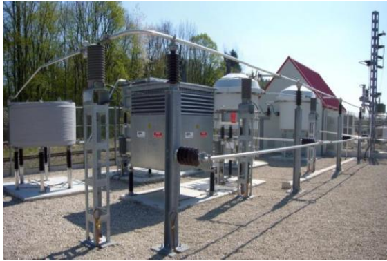
Outdoor equipment of a SVC
