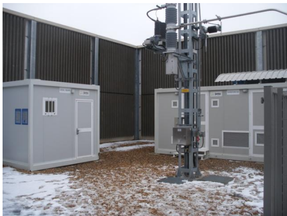
Outdoor equipment of a SVC
