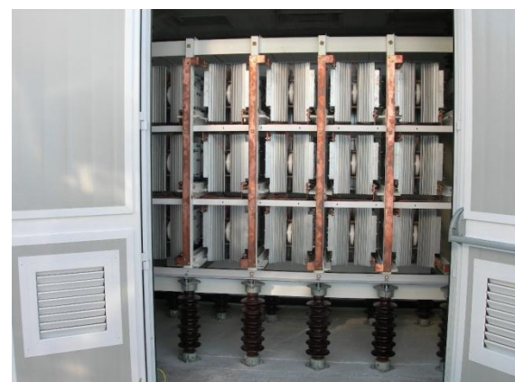
Natural air cooled valves in a container
